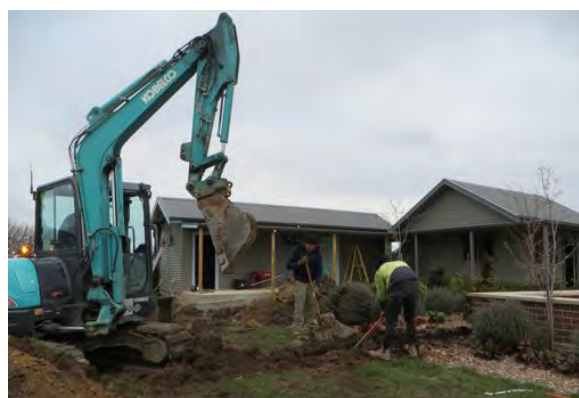
One of the coldest days in winter when John Barrett was supervising the installation of the drains
