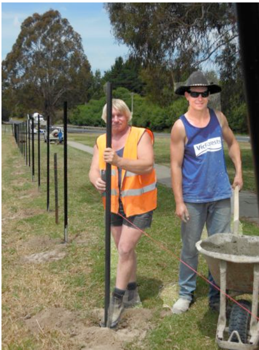
Contractor Greg Newman and his son Murray erecting the fence in November 2012
